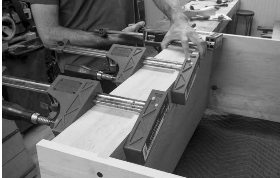
Long-grain kick. The kick is glued in place to the underside of the lower shelf. Then it is nailed in place through the sides of the bookcase.
